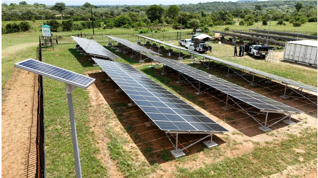
220KW Solar System in Chipinge
